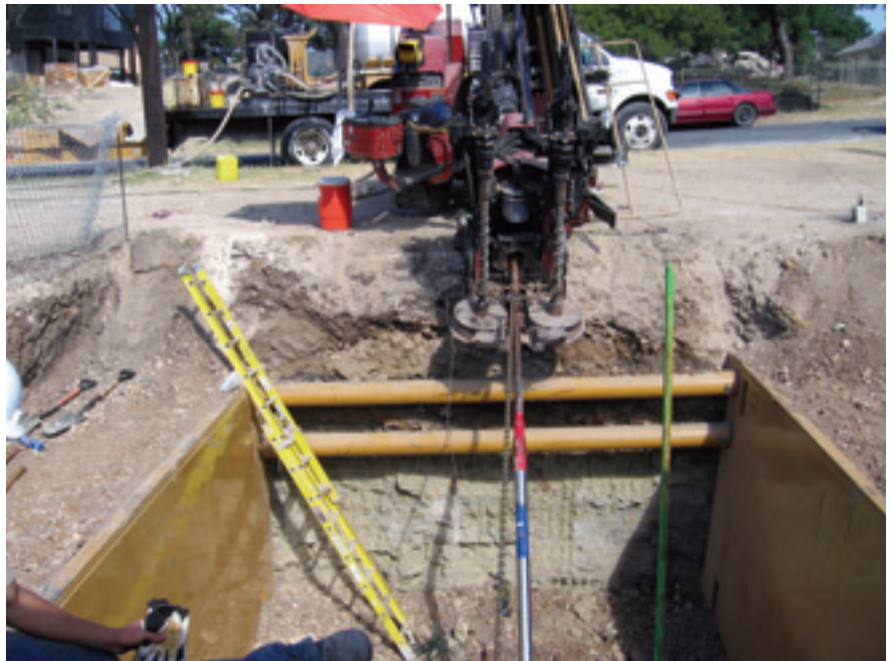
All three bores to the Shoal Creek tunnel were made with a compact Ditch Witch JT2720 All Terrain directional drilling unit.
