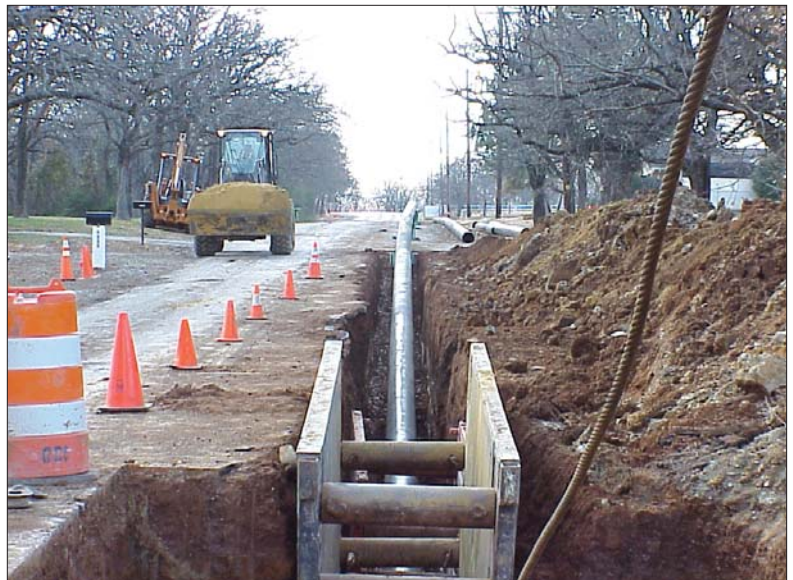
Planetary Utilities was hired to complete the HDD portion of a sanitary sewer project for the City of Fort Worth in which a rural-residential area was being connected to the City's sewer line. Eight-inch ductile iron pipe was installed inside 16-in. steel casing.
