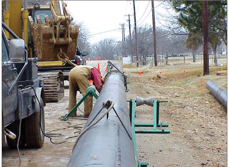
This project is believed to be the longest directional bore on grade for gravity sewers that’s been done. Total length, which was done in one shot, was 837 ft.
