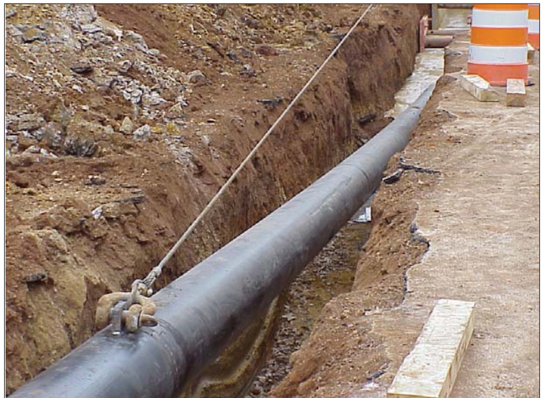
Among the challenges that the Planetary Utilities crew faced were the ground conditions. The crew drilled in mostly hard sandstone, which made it difficult to maintain pitch.
